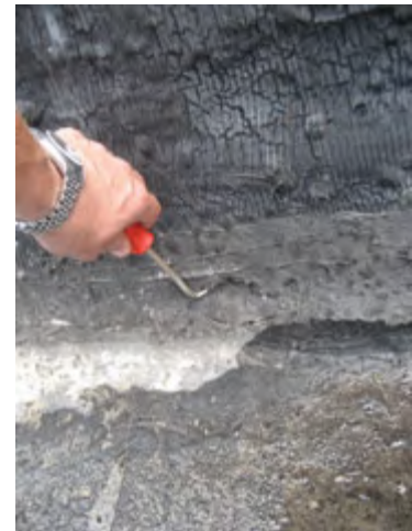
In this example, an existing roof has split plies at the base flashing, allowing water infiltration.
