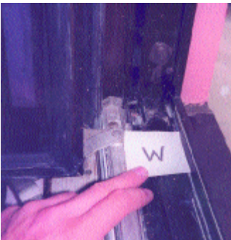
Figure 1: Shrinkage of poured-and-debridged thermal break at frame corner.
