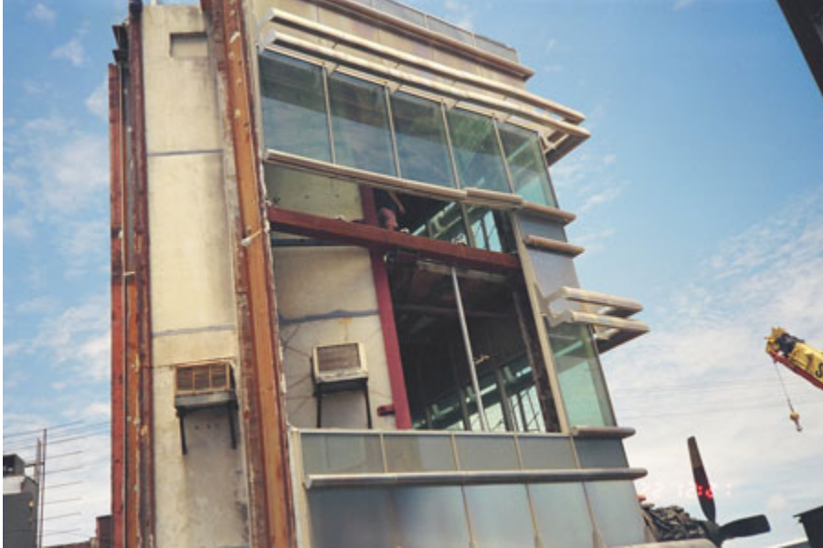
A recent mockup test found design and manufacturing flaws in this curtain wall system
