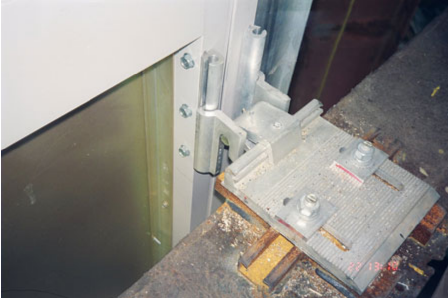
Movement of hooks off the pin observed on undamaged anchors.
