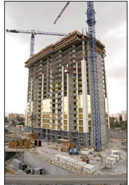
Construction continues on the first tower of the Residences at MGM Grand on May 10.
